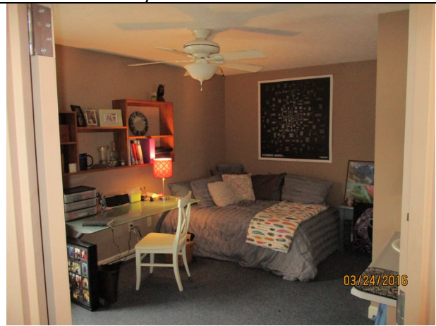
Ceiling Fans (in each Bedroom + Great Room)
